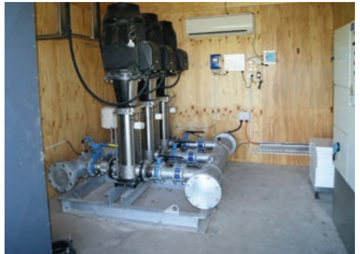
New pump shed
