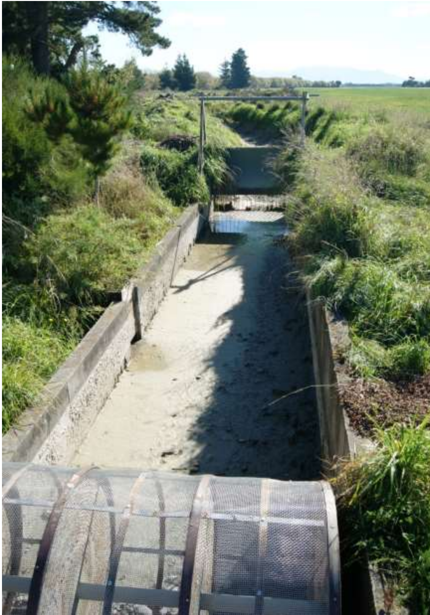
Figure 3-6: A view of the rotary drum at the Mead intake, looking upstream and without water flowing. The entrance to the fish bypass can be seen on the left side of the concrete channel.
