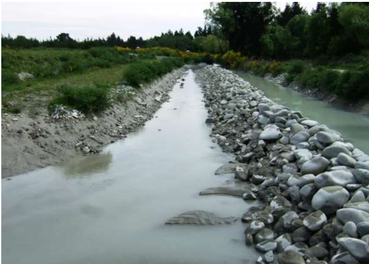
Figure 3-13: The permeable rock bund at the Acton intake, photographed looking upstream and with low supply channel water levels and scheme not operating (dewatered). The diversion channel supplying water can be seen to the right of the photograph, and the scheme intake channel to the left.
