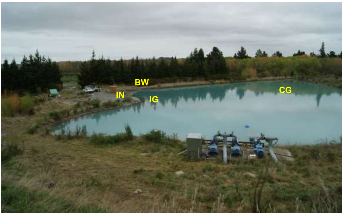
Figure 3-11: The SDC head pond. The infiltration galleries (IG) and SDC intake (IN) are situated near the vehicle seen on the left, and the bypass weir (BW) is on the edge of the pond to the right of the vehicle. In the foreground are the pumps for the Grasslands intake (not operating during this trial), and on the far right of the head pond is the control gate (CG) for water from the Rakaia River.
