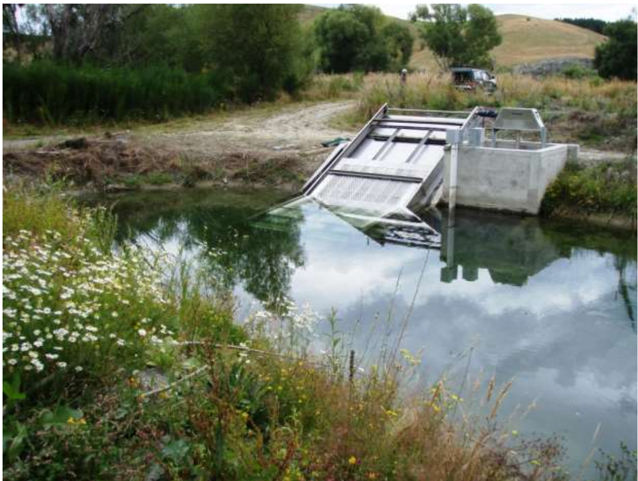
Figure 3-8: The ANDAR screen, on one side of the head pond. Water flows from the pond, through the screen and down into a channel behind the screen (adjacent to the parked vehicle).
