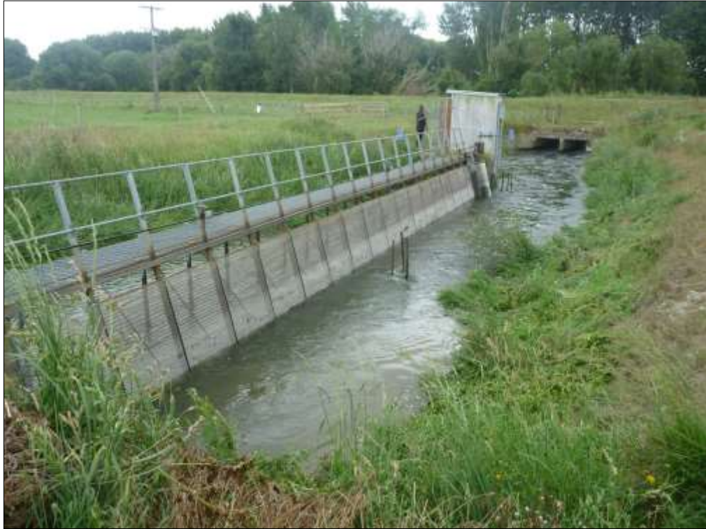
Figure 3-4: The Levels Plain intake screen. Water moving downstream (towards camera) passes through the screen panels and into the scheme intake channel behind the screens. The entrance to the bypass is under the vegetation at the bottom left. The stakes near the screen support the DIDSON camera used for the trials.
