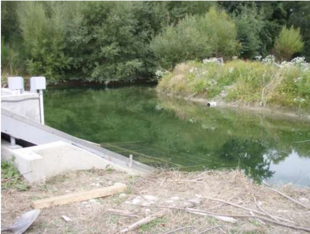
Figure 3-9: The bypass entrance; a pipe through the gravel bank opposite the screen. Water flows through the pipe into a small open channel that returns water to the Opihi River.
