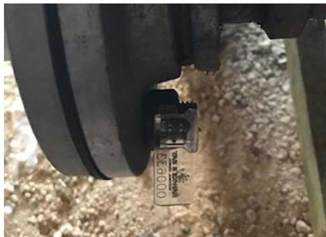
Image: An example of a Tamper Tag with a unique serial number inserted onto a bolt securing a flange.
