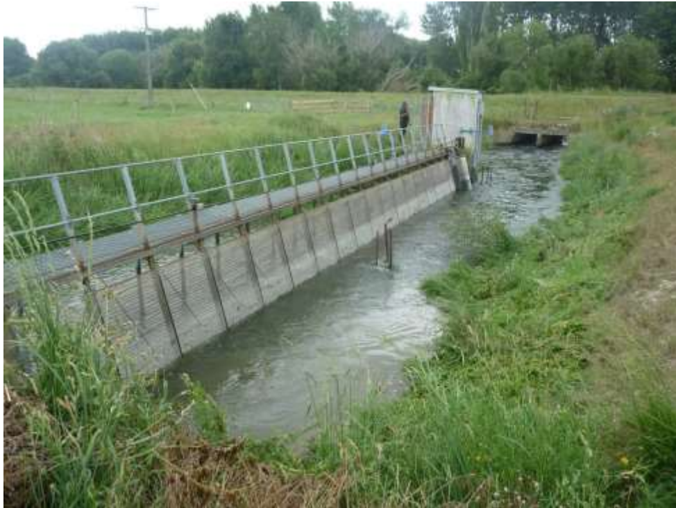
Figure 1: Level Plains Fish Screen (looking upstream)
