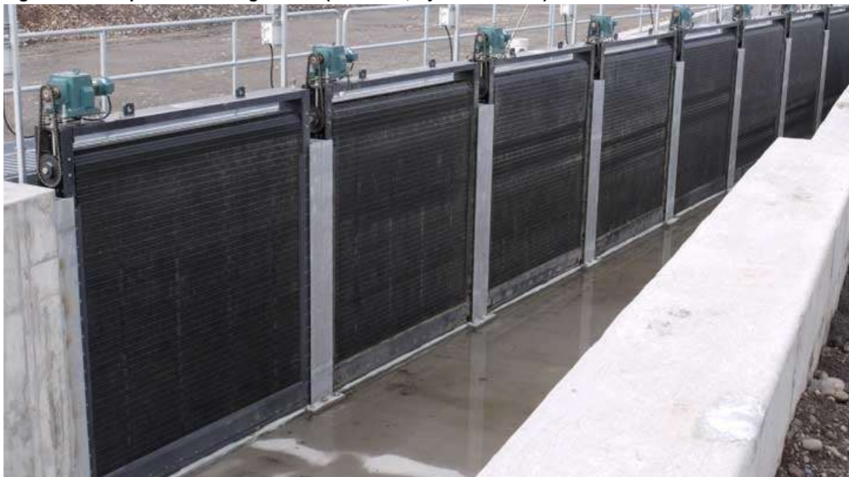
Figure 9: Example of Travelling Screen (Fall River, Hydolox Screen)
