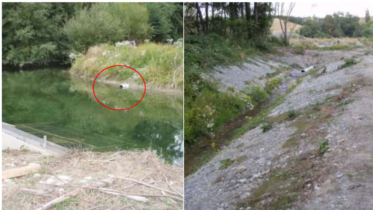
Photostat 1: Fish Bypass pipe inlet (left) and Fish Bypass pipe outlet into channel (right)
