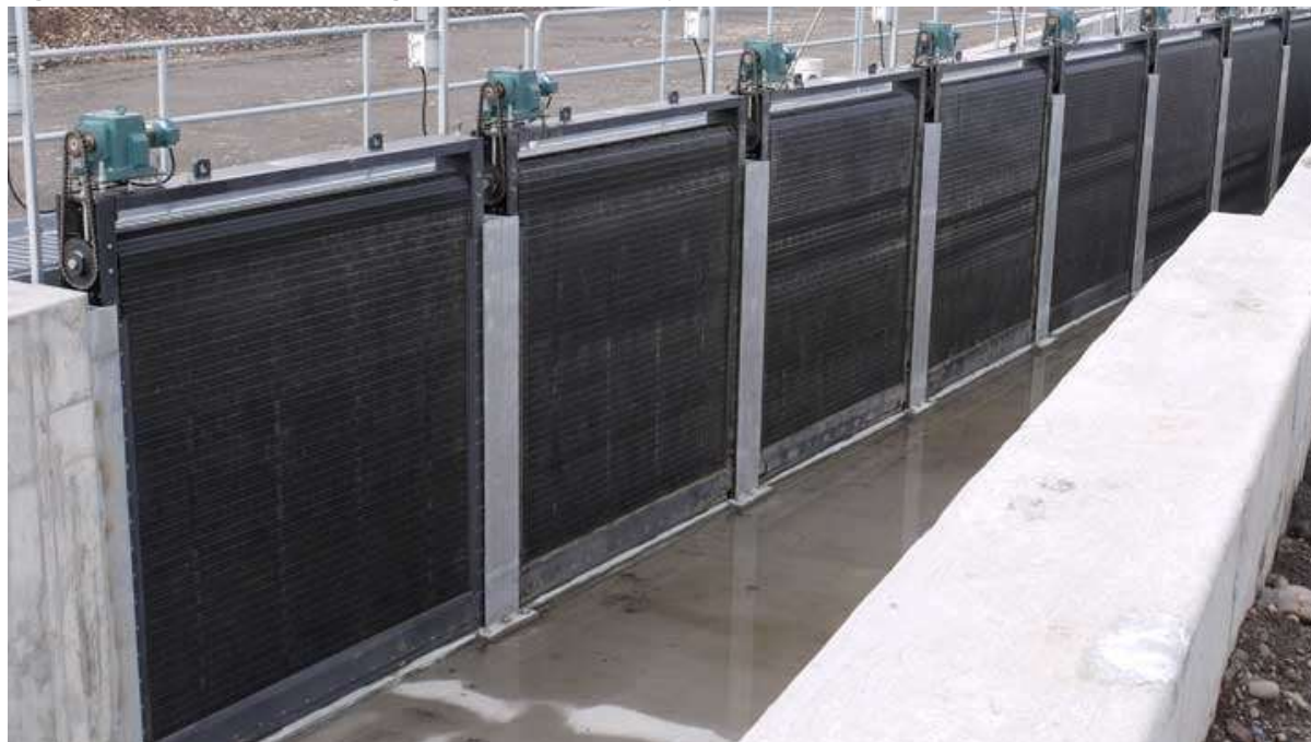
Figure 6: Example of Travelling Screen (Fall River, Hydolox Screen)
