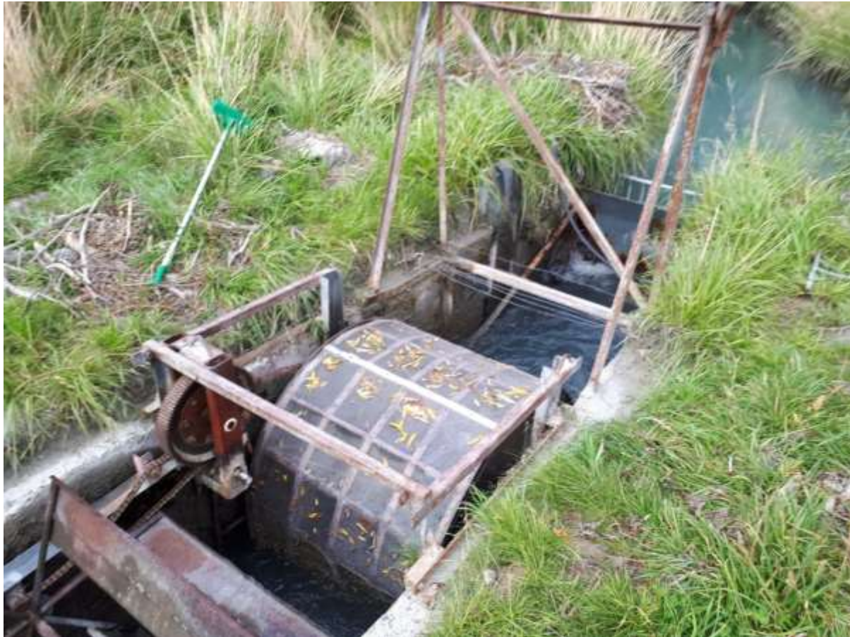
Photo 1: Existing Fish Screen
