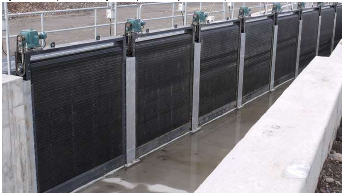
Figure 10: Example of Travelling Screen (Fall River, Hydolox Screen)
